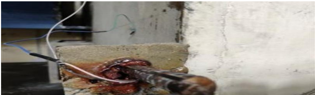
Figure 8: Image shows a reinforced concrete beam after corrosion.
